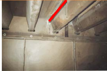
1. Possible fatigue crack in trough bridge
